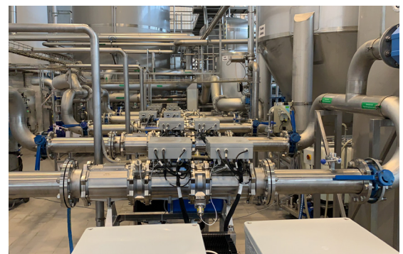
HOD™ UV provides product water disinfection and ozone destruction, reduces maintenance and operating costs at PepsiCo Domodedovo, Russia.
